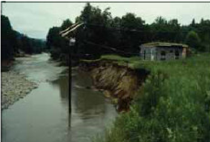
Fluvial erosion along the Mad River, Waitsfield, Vermont. Image courtesy of VTDEC River Management Program.
